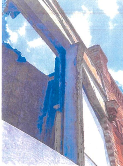
Leaning Beam Beside 8 Ball
